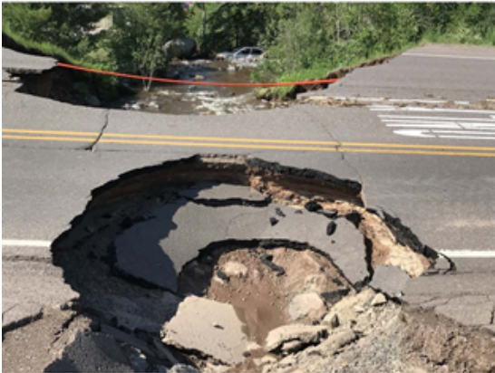
Failed pavement caused by washout in Houghton County, 2018 Photo: John Moore WSMH
