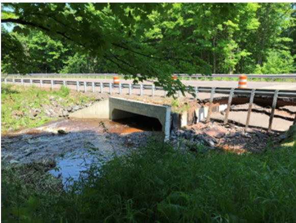
Box Culvert remained in place, partial roadway washout. Backfilled and reopened to traffic within 36-hours. Houghton County, MI 2018
