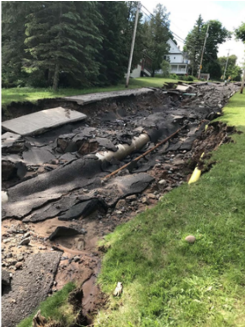
Concrete pipeline left in place after roadway washed out, 2018
