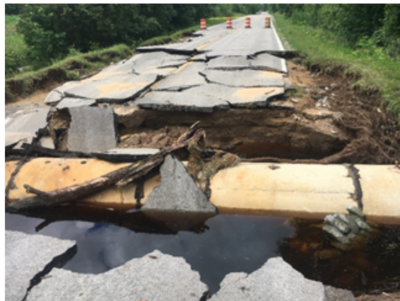
Concrete pipe remained in place following road washout in Bay County, MI 2017
