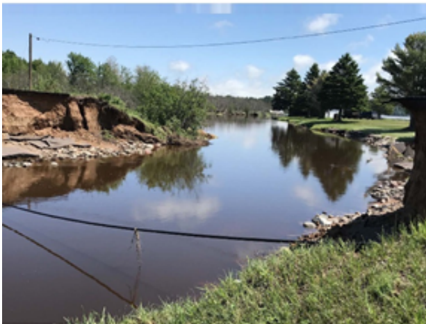
Washed out corrugated metal culvert. Houghton County MI, 2018
