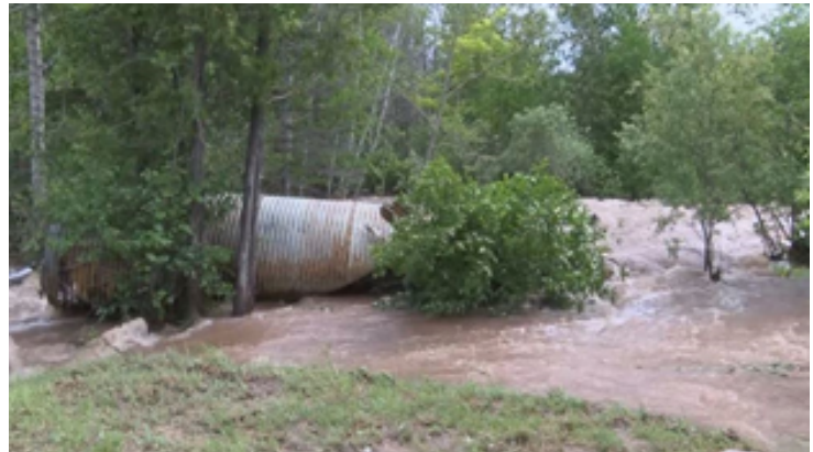
Washed out corrugated metal pipe, Houghton County, 2018 Photo: John Moore WSMH
