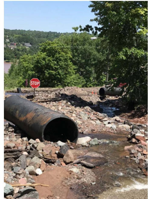
Plastic pipe washed out, Houghton County MI, 2018
